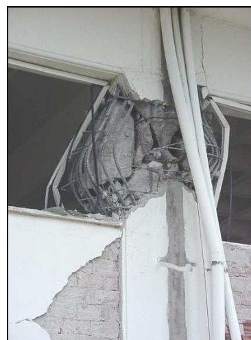
Fig. 1. Short (captive) column damage because of masonry walls not extending at full height of the column (1999 Athens, Greece, earthquake of 5.9 M)
