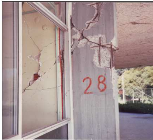
Fig. 9. Damage of RC column caused by failure of the adjacent masonry infill (city of Kalamata, Greece, at the earthquake of 6.2M, in September 1986)
