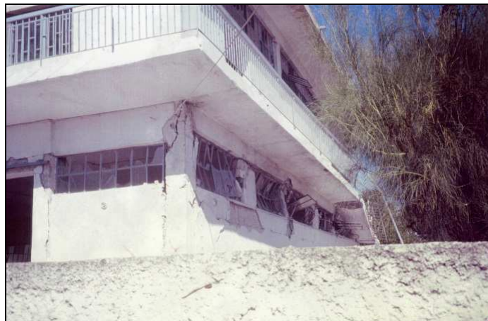
Fig. 2. Building collapse due to the existence of short columns (1999 Athens, Greece, earthquake of 5.9M)
